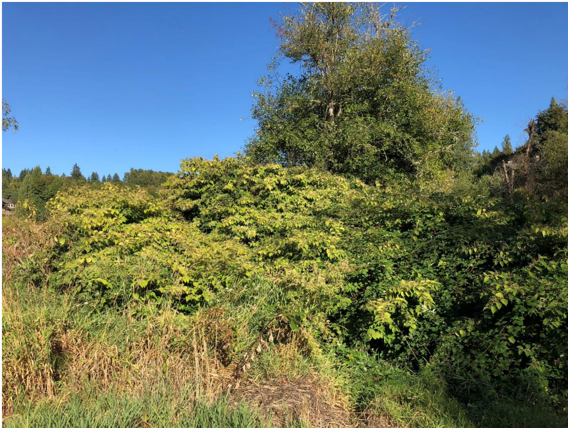
Lake Outlet overgrown with knotweed and blackberry, restricting access to spillway.
